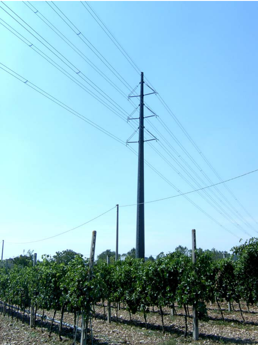
Bonomi's braced insulated cantilevers on some Terna's trellis in Italy
